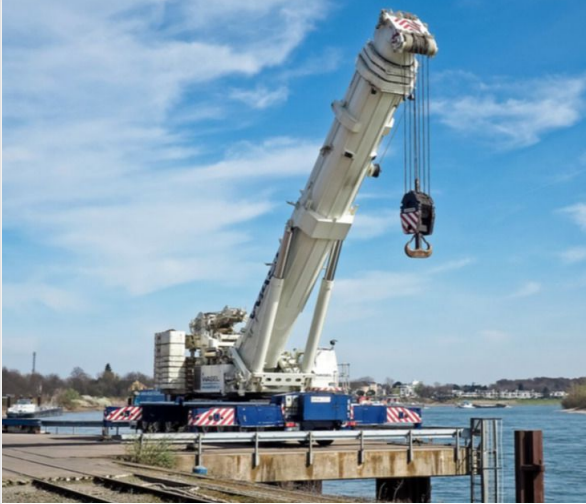
Crane with pulley block
