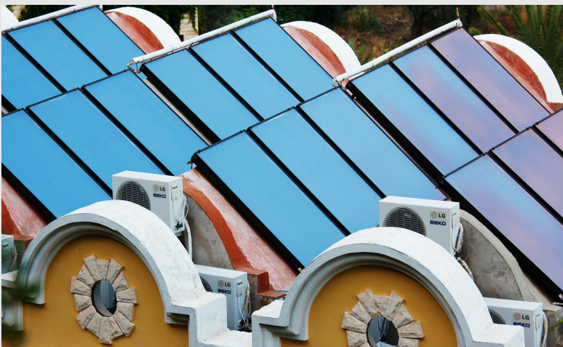
Solar thermal panels
