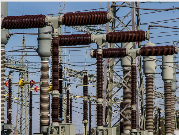
Transformers in a transformer station
