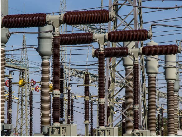
Transformers in a transformer station
